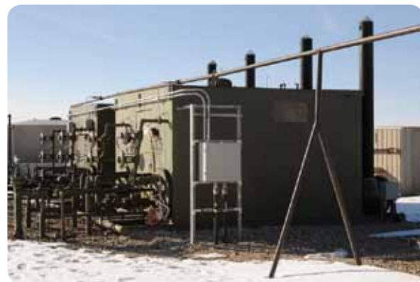
Count the stacks, each represents a well on a pad. These separator units remove the gas from the water coming from the well.
