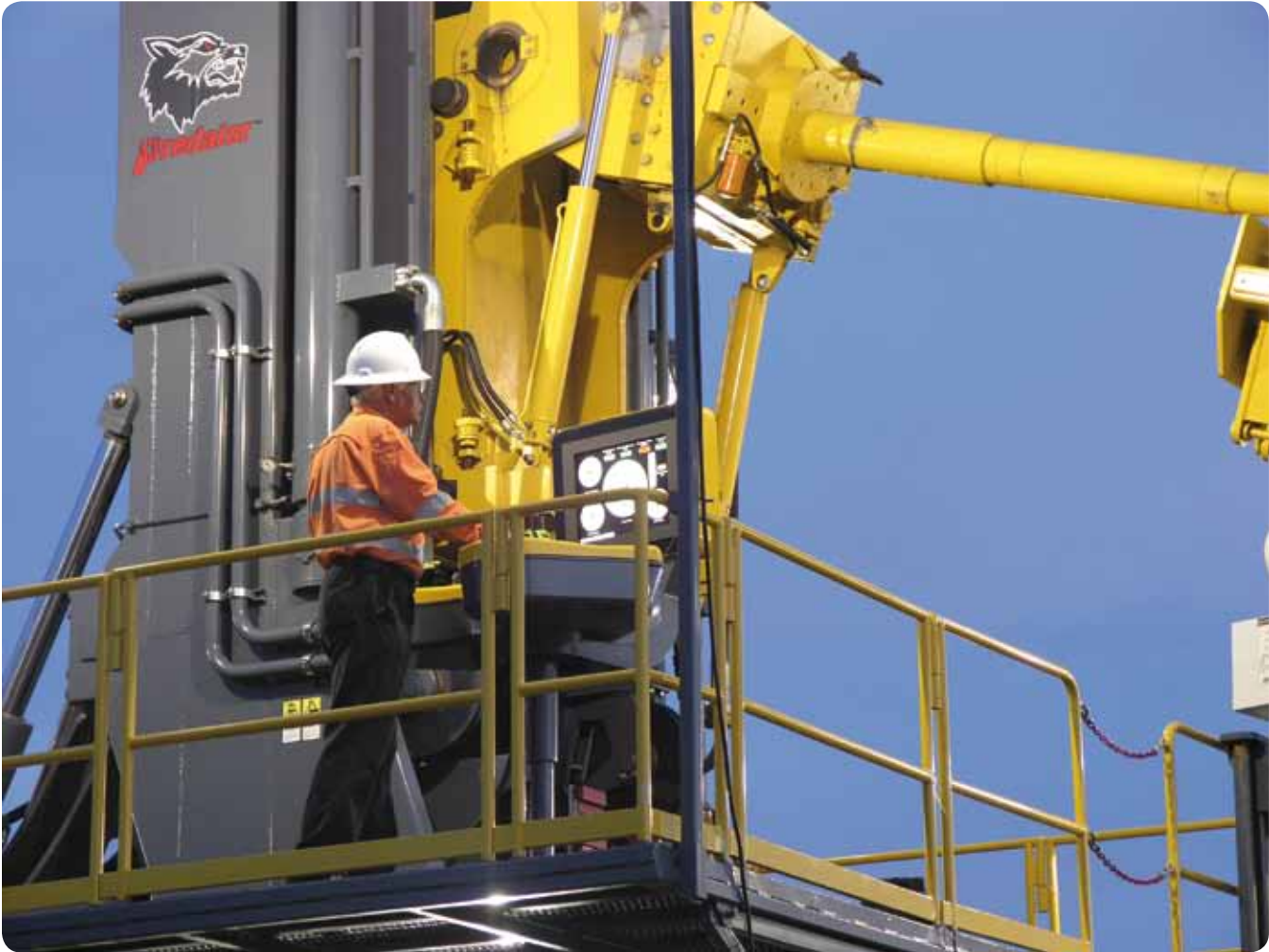
The drill operates with one man on the platform. All drilling functions and handling of pipe is done from the driller's station.
