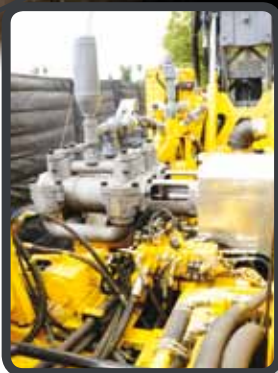
Clean working deck space with open access for maintenance.
