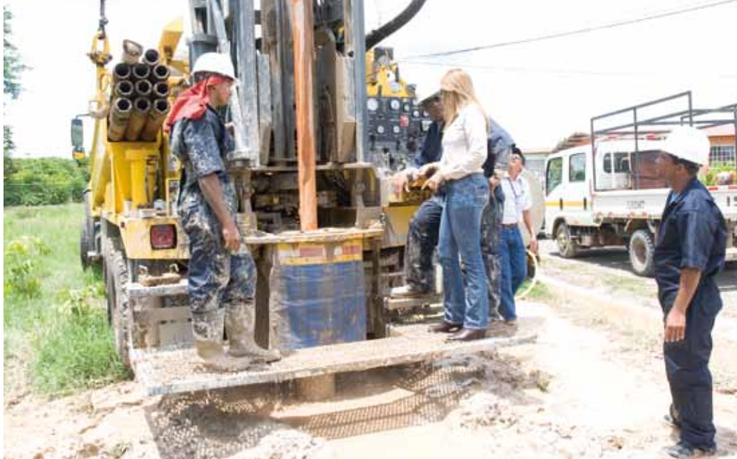
Workers near completion of the numerous wells of an IDAAN initiative to supply clean drinking water to all communities in Panama. Geology throughout the area required both mud and air drilling methods to penetrate the various layers of heavy loam and clay, consolidated sandstone and igneous rock.
