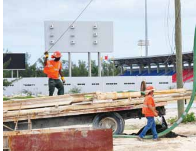
Drainage holes are for control of the rain water in parking lots and a future roadway for a large sports complex that's currently under construction.
