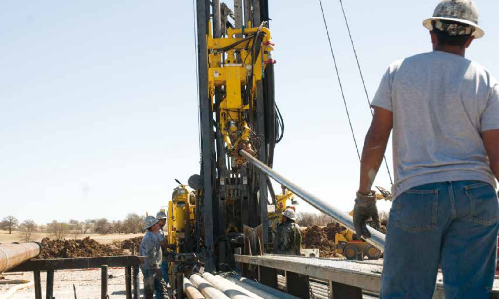
This Atlas Copco file photo shows the ease of pipe handling with the RD20 XC.
