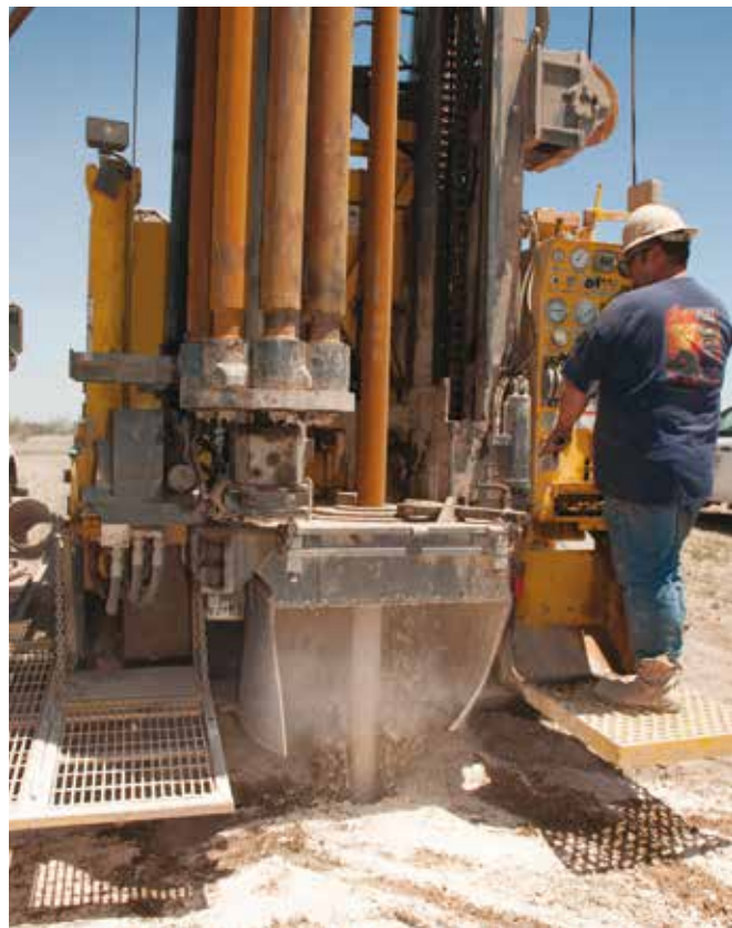
About 80 percent of the wells drilled in this part of the University Lands will lose circulation somewhere after 300 feet. THI drills with PDCs on air, misting three gallons a minute until that point. Then they will switch to 200 gallons of clear water per minute, none of which they’ll see return.
