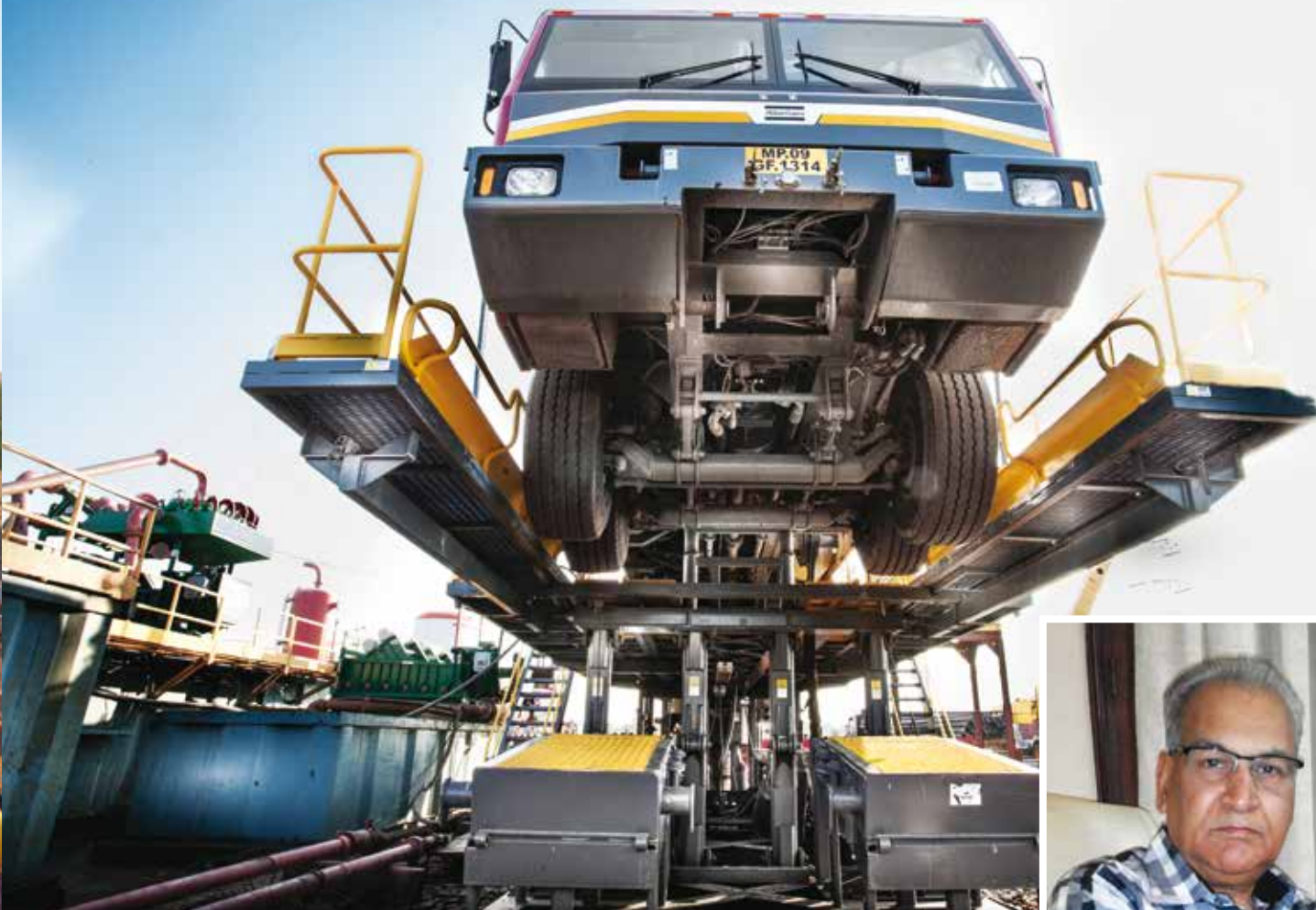
Using the Predator Drilling System, Shivganga Drillers Pvt Ltd. was able to drill more than 1,300 feet (400 m) in 18 hours, which they believe to be a record under these conditions.
