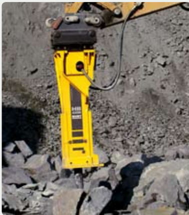
Good breaking: The HB 4200 hydraulic breaker in action. Mounted on a Cat 345 hydraulic excavator, the breaker is used either for breaking oversize blasted rock or for clearing rock-jams in the crusher.
