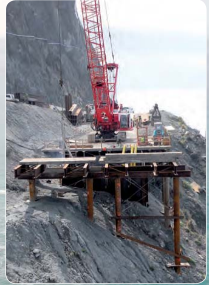
A wide angle view of the work site shows the coffer dam, trestle and Atlas Copco XAS 1600 compressors.
