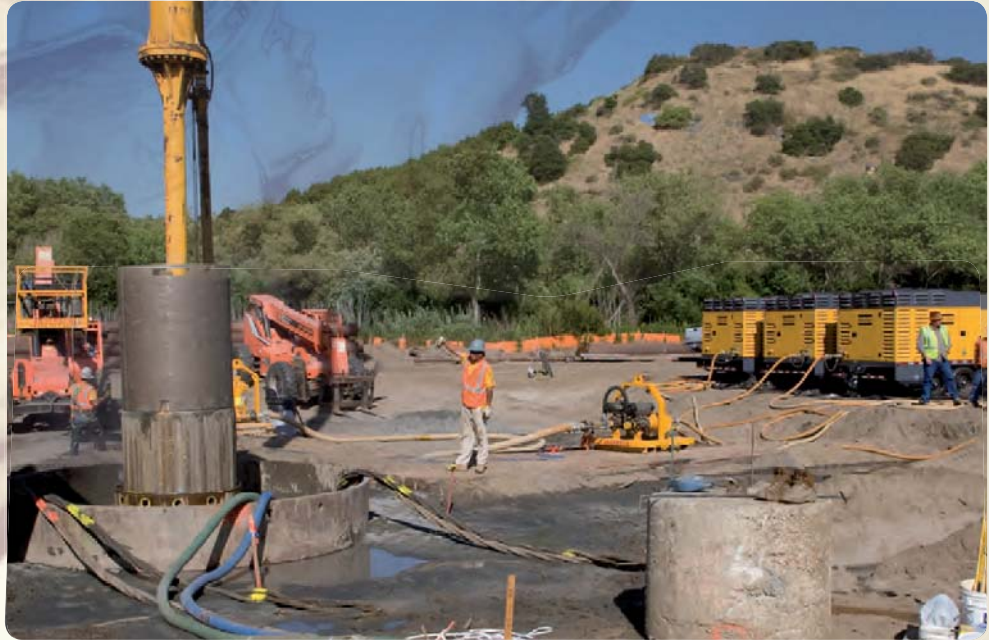
Along with the 48-inch cluster drill, three Atlas Copco XAS 1600 CD6 compressors were vital pieces of equipment on this job site.
