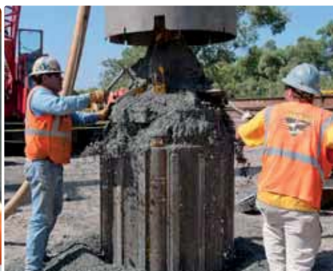
Emptying the Calyx basket: It takes about 20 minutes to lift the drill, remove the cuttings and return the drill to the hole.
