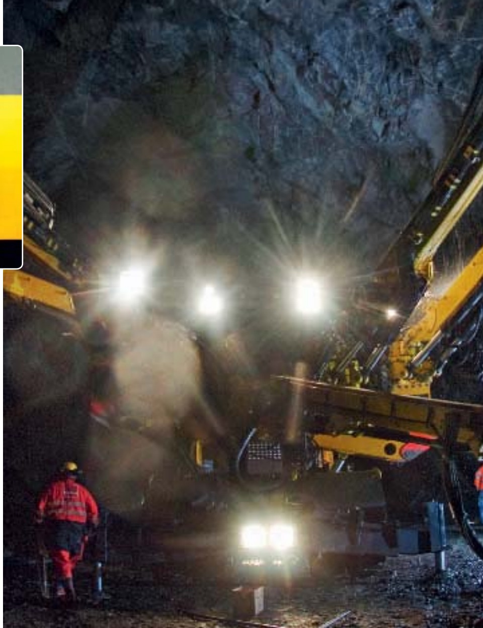
Inside the Kattleberg mountain: The fully computerized Atlas Copco Boomer XE4 C drill rig drills blast holes as well as pre-grouting holes in what will be the new rail tunnel.
