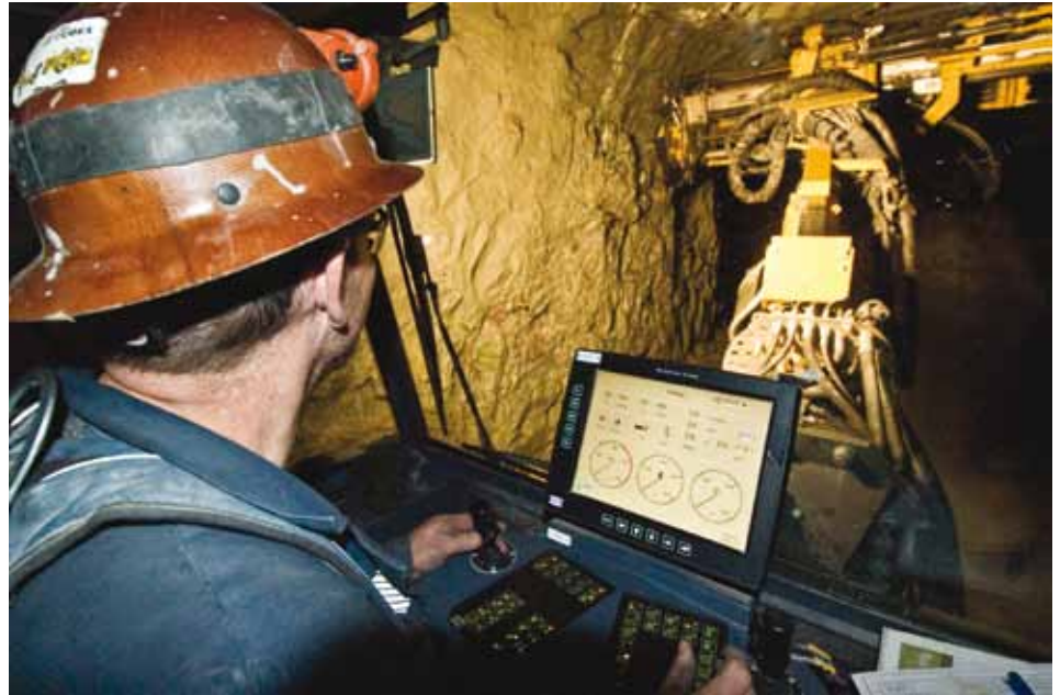
In the Simba M7C the operator sets up the rig to drill holes at any angle in perfect placement. Most of the time this Simba is drilling vertically to accommodate long hole stopeing, but here the operator is drilling 5-inch diameter holes from one drift to another to run electrical lines.
