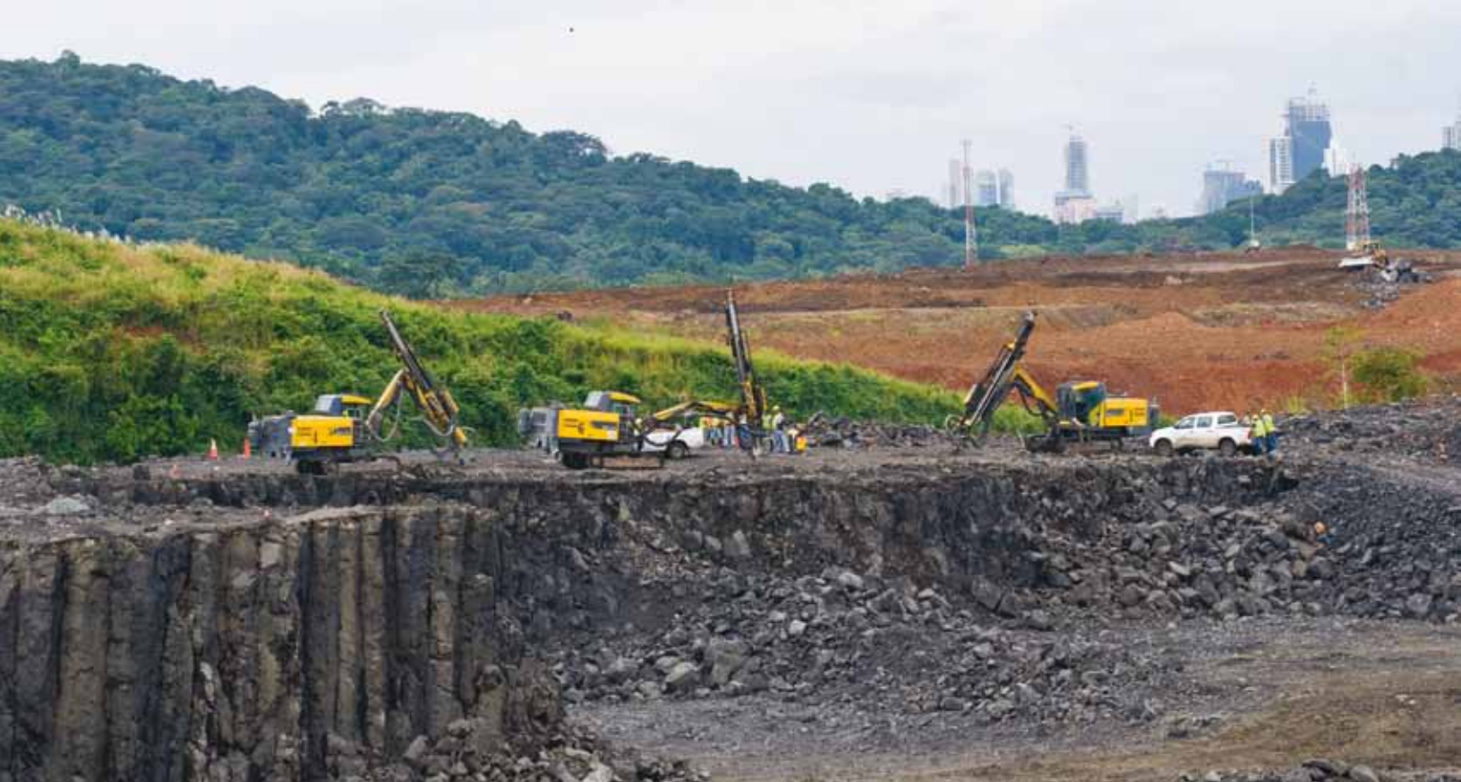
Atlas Copco's ROC D7 is the drill rig work horse on the Panama Canal expansion project. Panama City high-rises can be seen in the distance.
