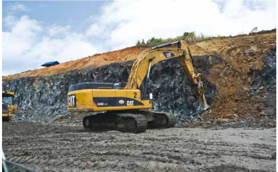
Panama: The Atlas Copco HB 3000 Hydraulic Breaker is not part of mining production, but very necessary to keep the shape of the canal wall. Voids and unconsolidated rock will cause poor blast areas.
