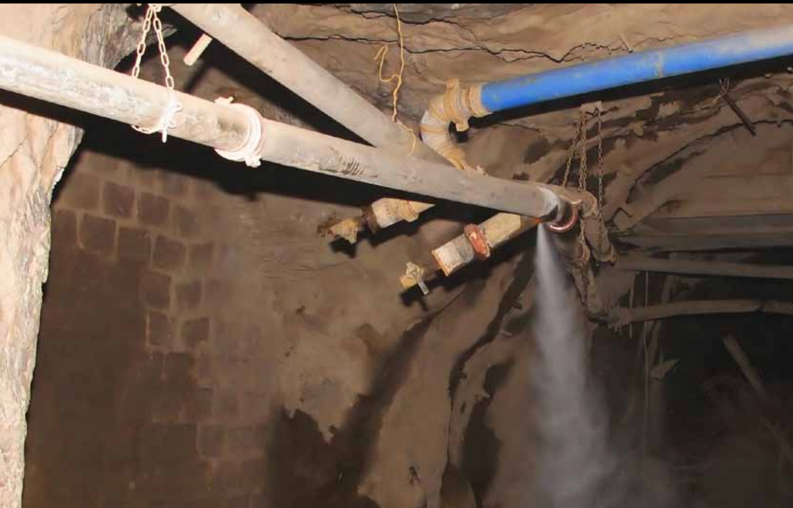
Leaking money: Compressed air pipelines that sometimes run for several kilometers in a mine are usually bolted together every five metres with a subsequent risk of leakage from the joints. The longer the pipeline, the greater the risk. Even the best systems can lose about 30 percent says Lars Bergkvist.
