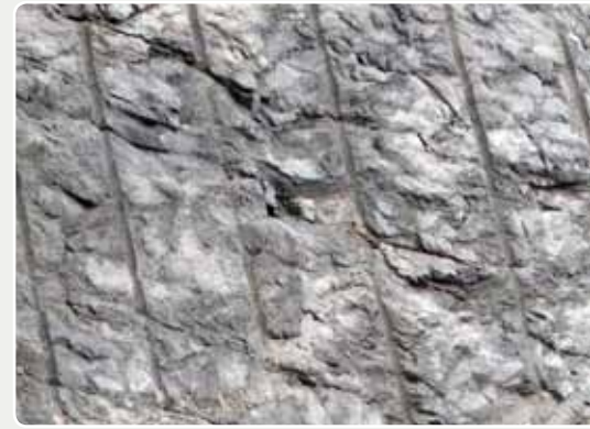
Visible evidence: The fact that the drill hole marks can be clearly seen proves that presplitting has been properly executed with closely spaced, straight and parallel holes, blasted with light charges ahead of the buffer and production holes.
