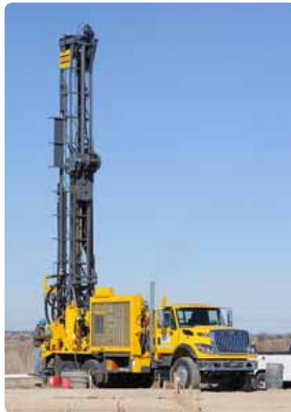
Geothermal drilling in Finland: Atlas Copco already has a range of suitable products and the necessary know-how to make a substantial contribution.
