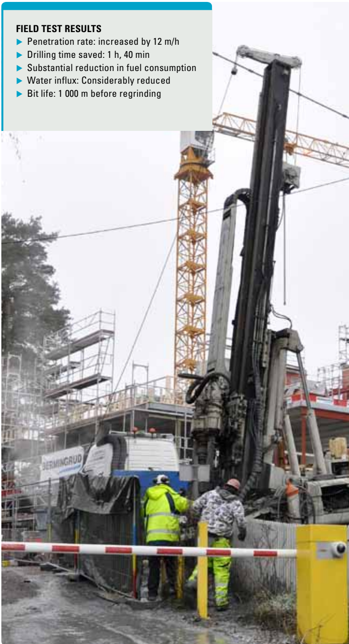
Putting EDGE to the test: Here the equipment is used in the drilling of nine, 500 m deep holes for a major apartment complex near Oslo.
