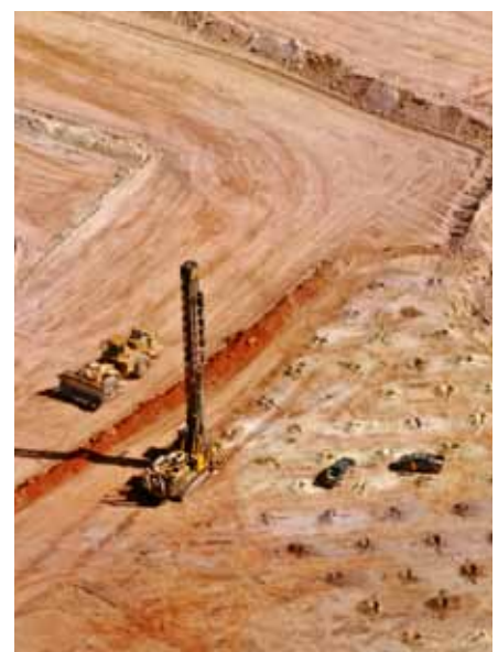
View from the top: The Pit Viper 271 working the 15 m high benches at Veladero.
