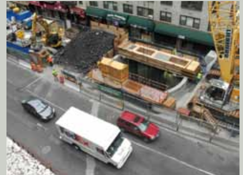
Phase 1 of the Second Avenue Subway includes a two-track line along Second Avenue from 96th Street to 63rd Street with a connection from Second Avenue through the 63rd Street tunnel to existing subway lines. The total project cost is $4.45 billion.
