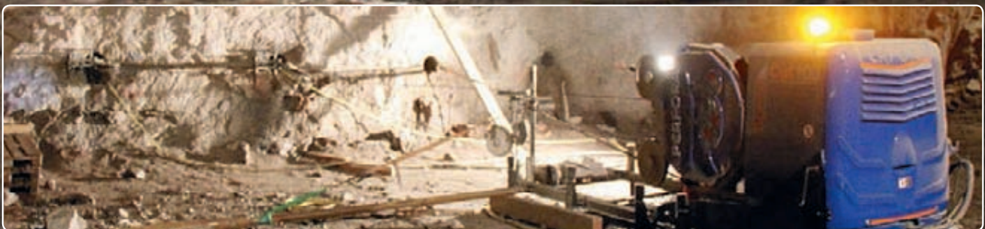
Keeping the peace in Stockholm: The SpeedCut saws out the rock to make way for a new subway tunnel without creating disturbing vibrations.
