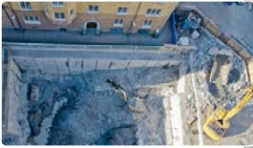
Keeping vibrations at bay: Protecting the nearby residential homes and, right, St Matthew's Church both just about one meter from the edge of the worksite.
