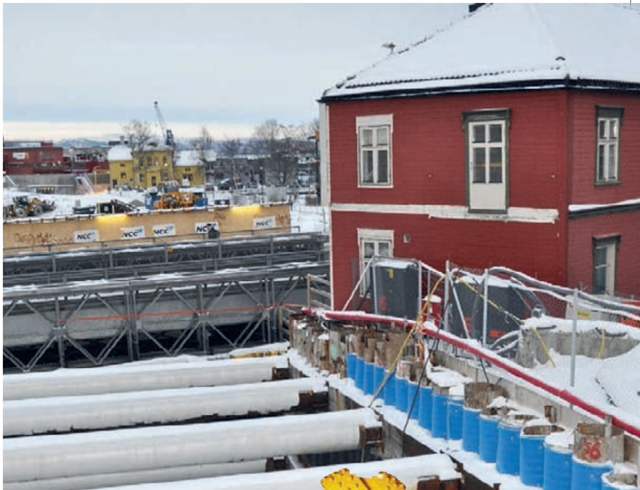
Too close for comfort: One of the buildings that were removed completely intact and later put back in exactly the same location.
