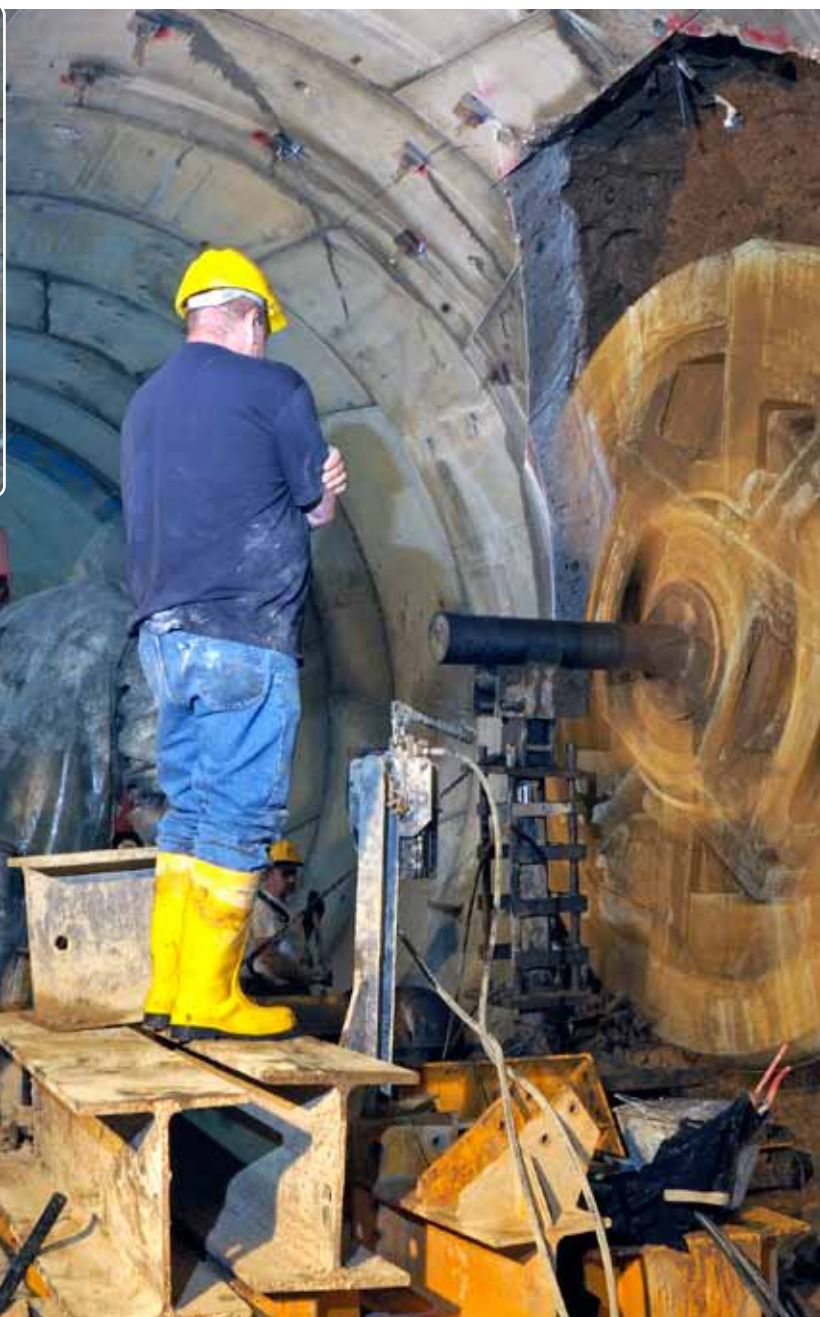
Raiseborer in action: Tunneling engineers use an Atlas Copco Robbins 53RH raiseborer machine to install a series of openings that will relieve the air pressure inside the new subway that runs 30-40 m below the city of Naples. Top left, a completed opening.
