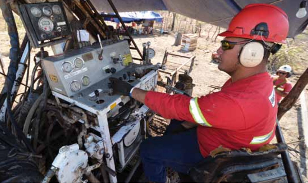
Rodio mounts the drillers station above the drill area giving the operator clear view of the work area and winch lines.
