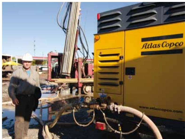
Stanley Reitsma stands next to the Atlas Copco XRVS 1000 CD6 compressor that is providing air to two drill rigs.
