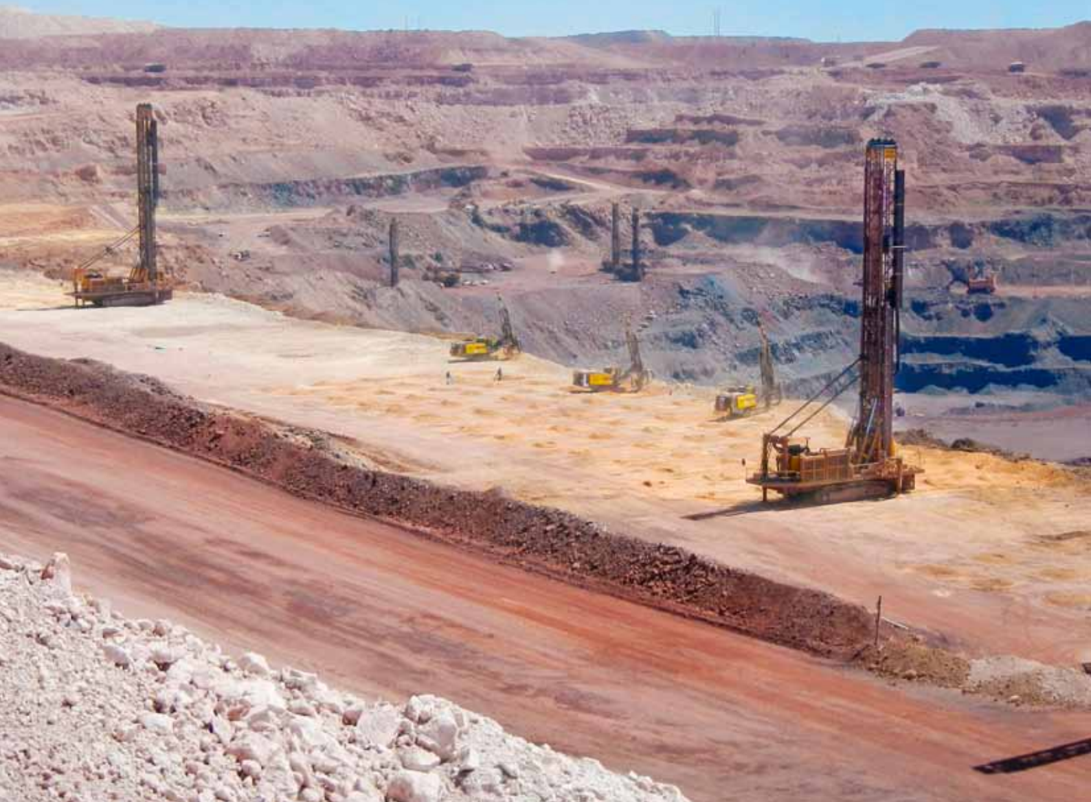
Overview of the massive iron ore mine at Sishen: Pit Viper 351 rigs drill the blastholes while ROC L8 rigs take care of crest drilling at the Sishen mine.
