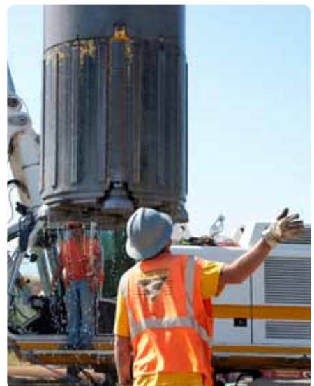
...and a cluster drill consisting of seven hammers for tunnel foundation work in the USA.
