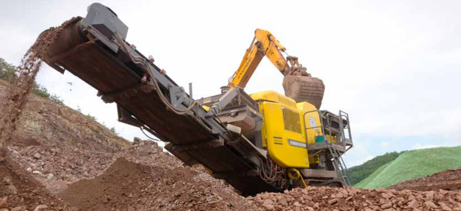
Recycling for sustainability: Here, the impact crusher Powercrusher PC 3 is used by Samwoo Recon at Chilwon to recycle road construction material into new base stone.
