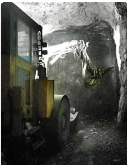
A safe alternative: The Scaletec rig, now routinely used at Tara Mines for scaling.
