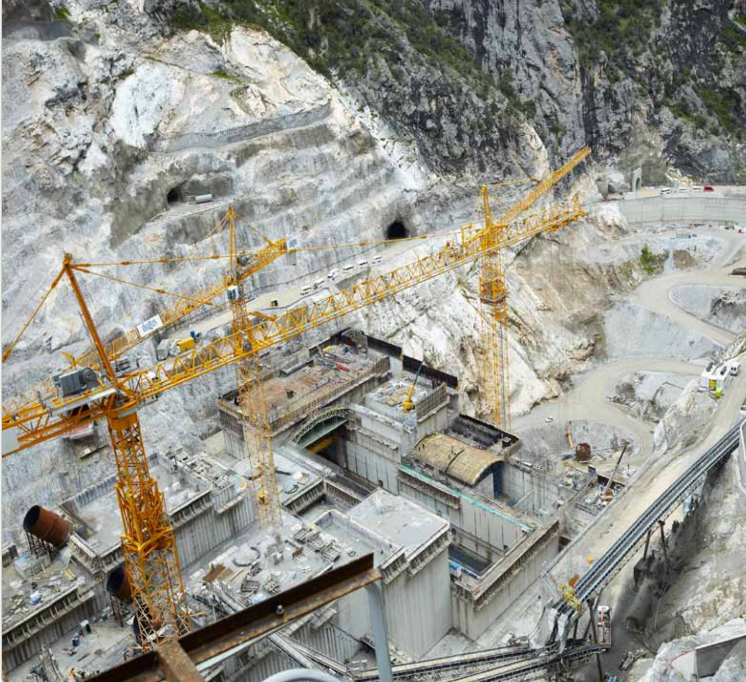
A grouting mega-challenge: This extensive project to seal and stabilize the Boyabat Dam was part of a construction record that puts Turkey on the path toward far-reaching hydropowered energy.
