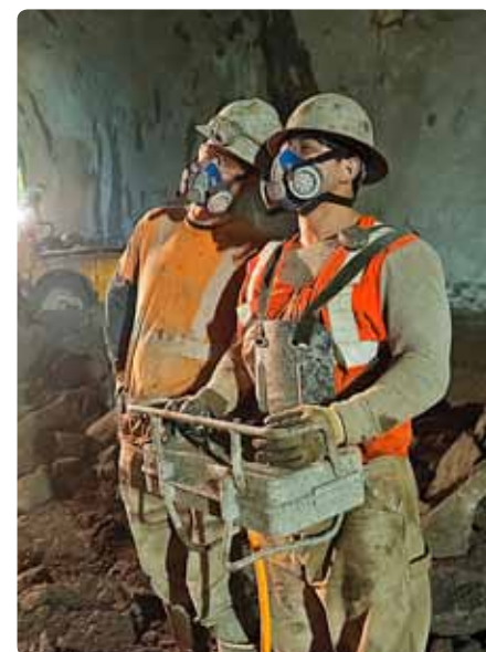
Total concentration: MEYCO operators apply the final layer of shotcrete to a wall using the Suprema machine's remote control.
