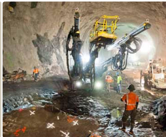
Setting up: The Boomer E2 C during the drilling of the cavern's top heading.
