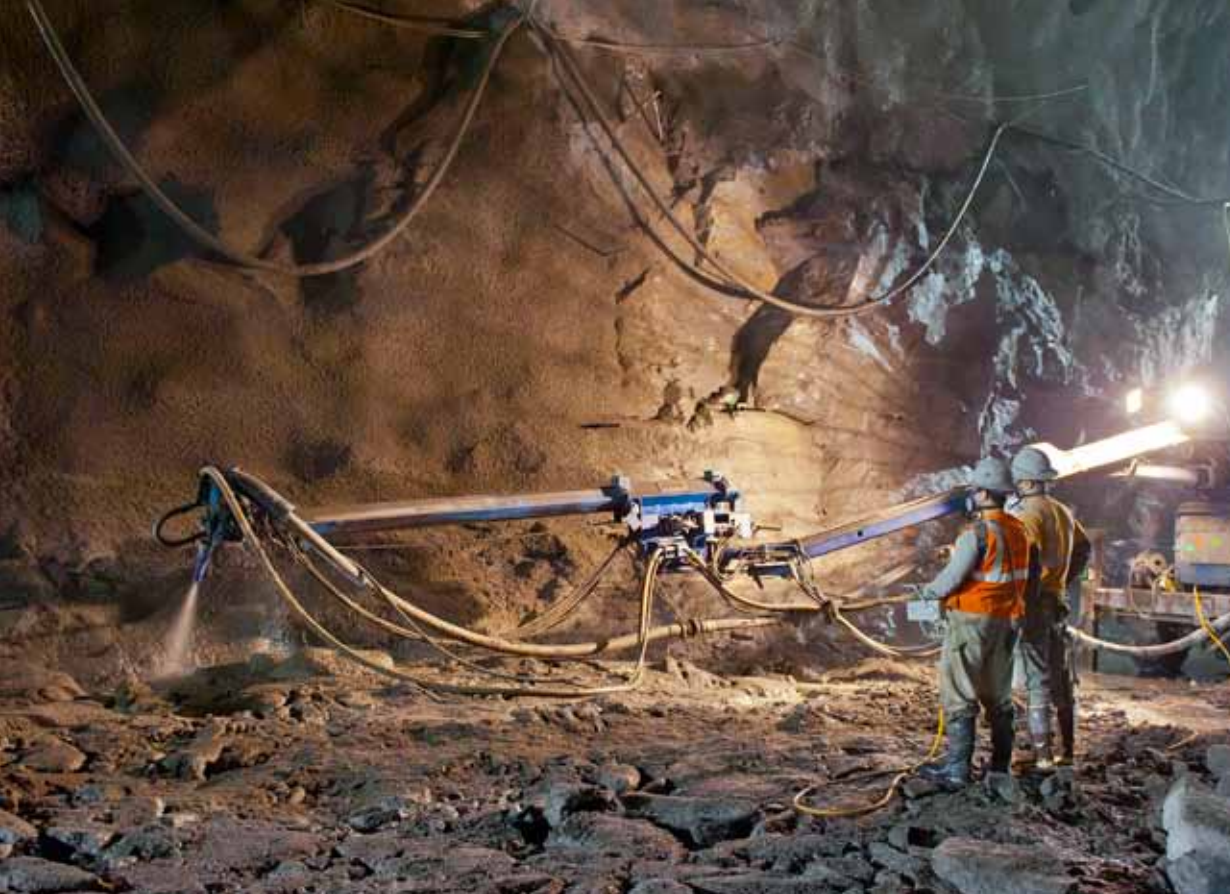
Reinforcing the rock: Using Atlas Copco MEYCO's Suprema spraying equipment, three layers of shotcrete were applied, two layers of a fiber reinforced mix including a superplasticizer, before and after bolting, plus a third non-fiber coating prior to the installation of a PVC water membrane. Together, the layers formed a minimum thickness of 250 mm overall.
