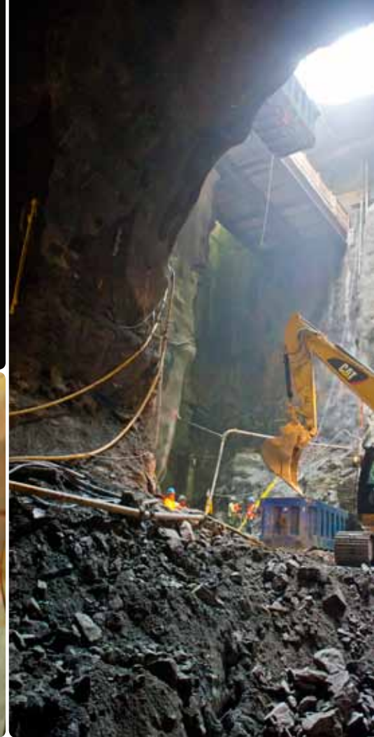
The only way is up: After blasting, all of the muck was hoisted to the surface in boxes at the rate of 700–1 000 tonnes per day.
