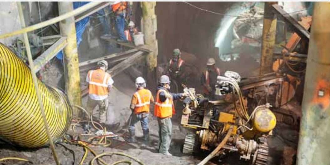
A major challenge: Workers set up the compact FlexiROC T30 in the access shaft at the north end of the 86th Street project.
