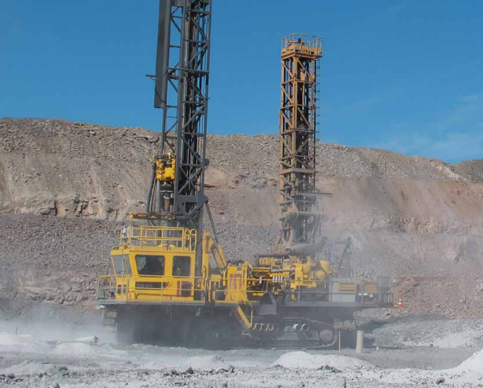
Single-pass to multi-pass drilling: The DM-M3 rigs arrived at the site in 2012 and can be used for single-pass drilling to depths of 12 m. Currently, these rigs are used for multi-pass drilling, using two 12.2 m pipes, to drill down to a depth of 21 m.
