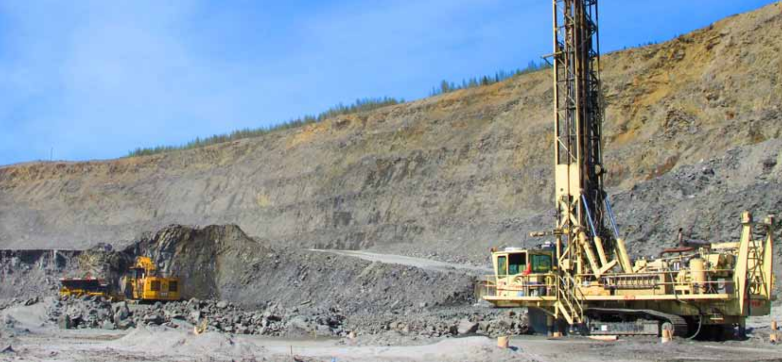
Tackling the hard stuff: A number of Atlas Copco Pit Viper 275 multi-pass blasthole drill rigs are also used in the pits and the mine recently took delivery of a new one which will be used in locations where the rock is exceptionally hard.
