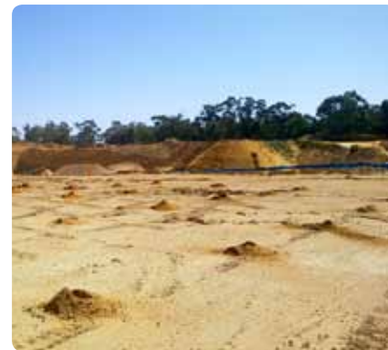
Job done! The completed drill pattern of 15 holes, three rows of five per row, after remote drilling with full automation.
