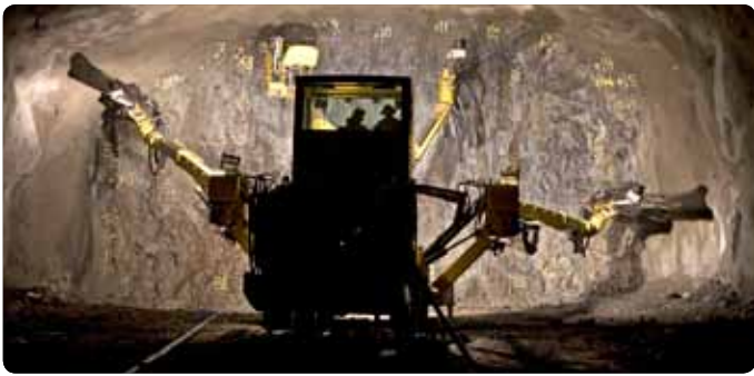
A powerful team: Six Boomer XE3 C drill rigs are at work on the new road-rail tunnel projects in Norway.
