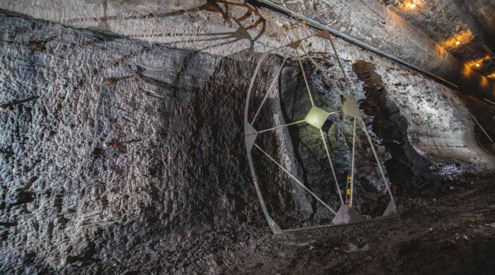
A special template was designed by Technicore to outline the profile shape on the tunnel.
