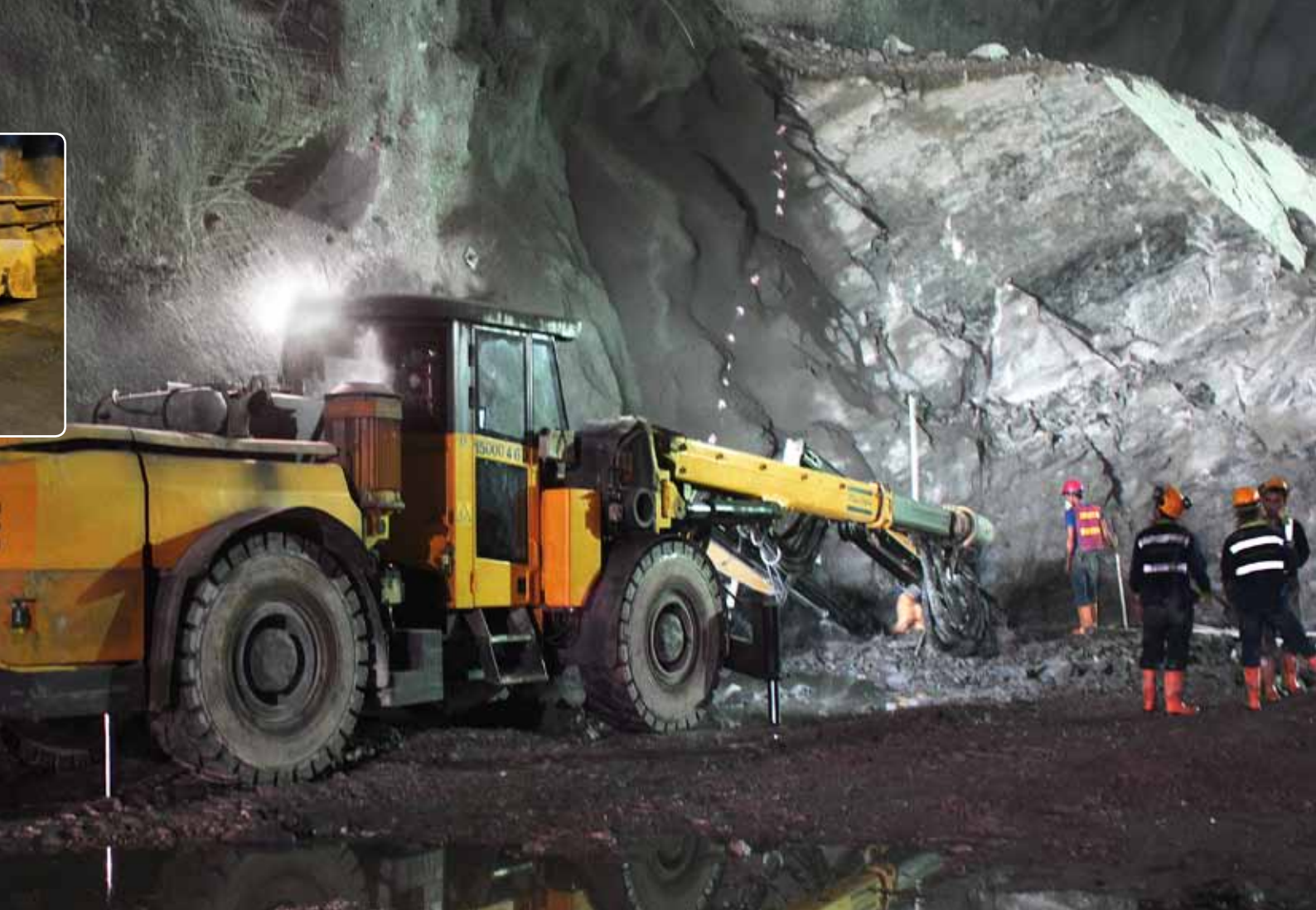
Paving the way for more energy: A two-boom Boomer E2 C drill rig from the Atlas Copco fleet excavating the tunnels and caverns at Ituango which will ultimately increase Colombia's electricity generating capacity by a further 2 400 MW.
