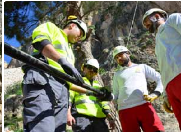
Atlas Copco's Deyvi Akkris and Bahadır Ergener, Sales Engineer and Business Line Manager, instruct the team on how to install the Swellex Pm24. Right, the APSP 300 Swellex pump is hoisted into position.
