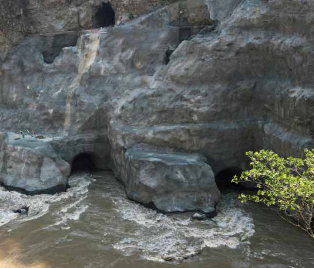
The power of the Cauca River: View of the tunnel portals of the temporary diversion intake tunnels.
