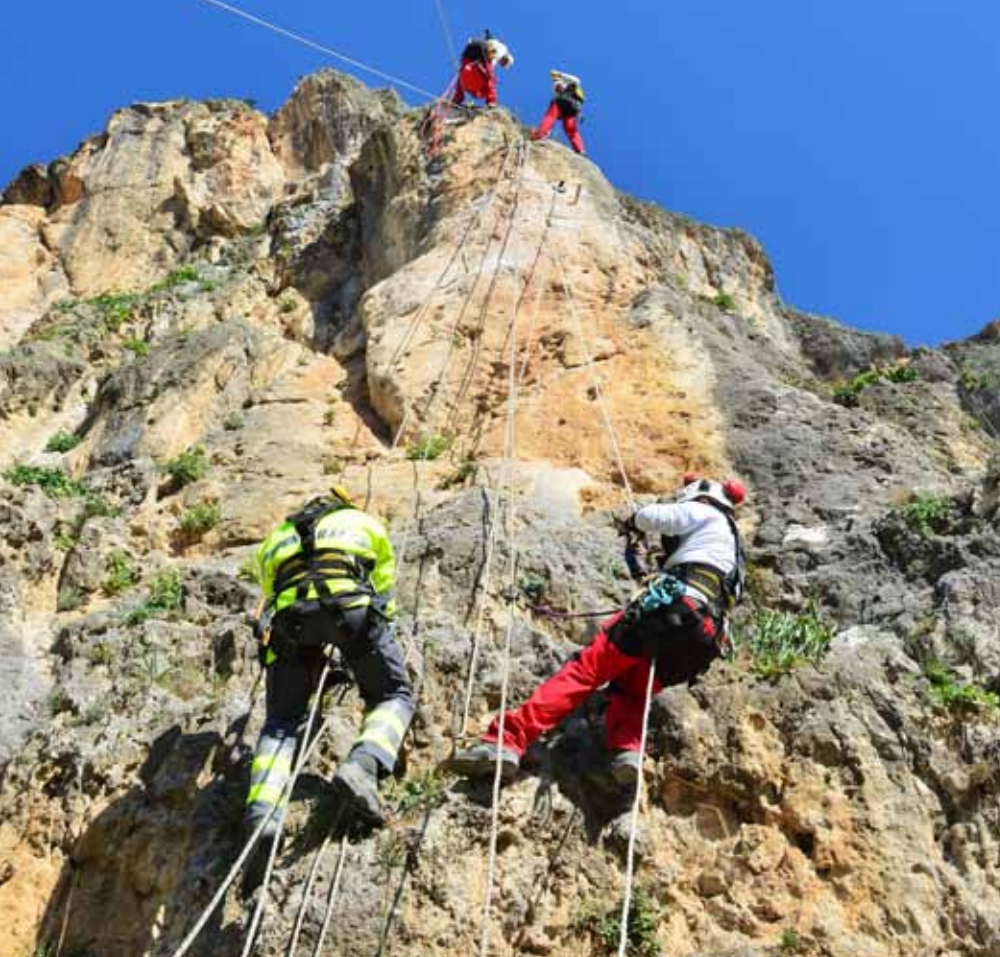
Swellex to the rescue: These mountaineers had to abseil down the mountainside to reach the section of loose and crumbly rock that threatened to fall on the famous cave church of St. Peter's.
