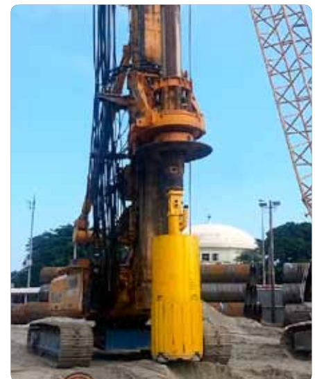
The cluster drill is lowered into position to start the first hole at the Rio Barra bridge.
