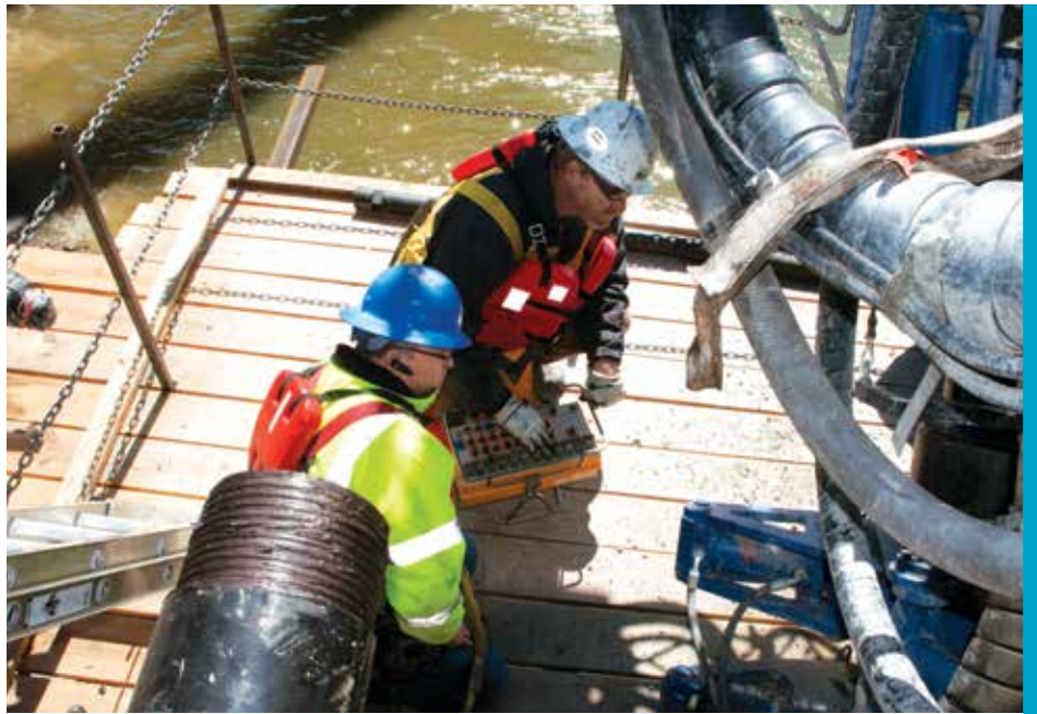
(above) Stacy Lynn, of the Atlas Copco–Nashville store, is on site as GeoFirma owner and driller Eric Snyder begins the first of three 105-foot anchors. The anchors consist of stranded cable grouted into a 20-foot rock socket in the Cumberland River Park Stabilization Project at the park’s scenic overlook.
