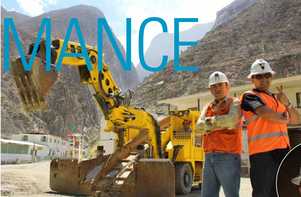
Outside the tunnel at the Quitaracsa hydro: Adan Nanquen and Oscar Parra with the Häggloader.
