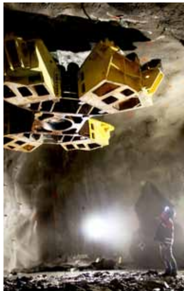
Going up! The huge cutter head on the Robbins 91RH reams up the pilot hole.
