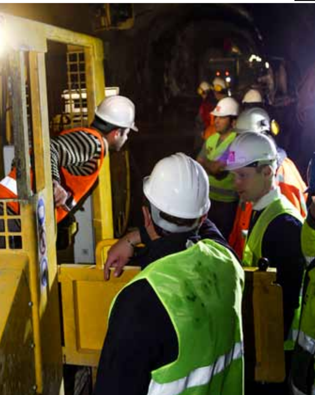
Inside the tunnel: Above, the team discusses the optimum setup in the confined space at the face.
