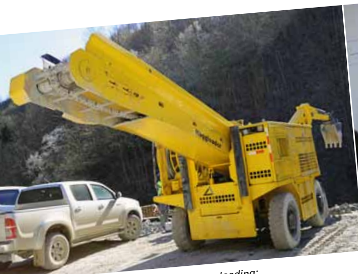
Essential equipment for continuous loading: The Atlas Copco Häggloader outside the entrance to one of the diversion tunnels.
