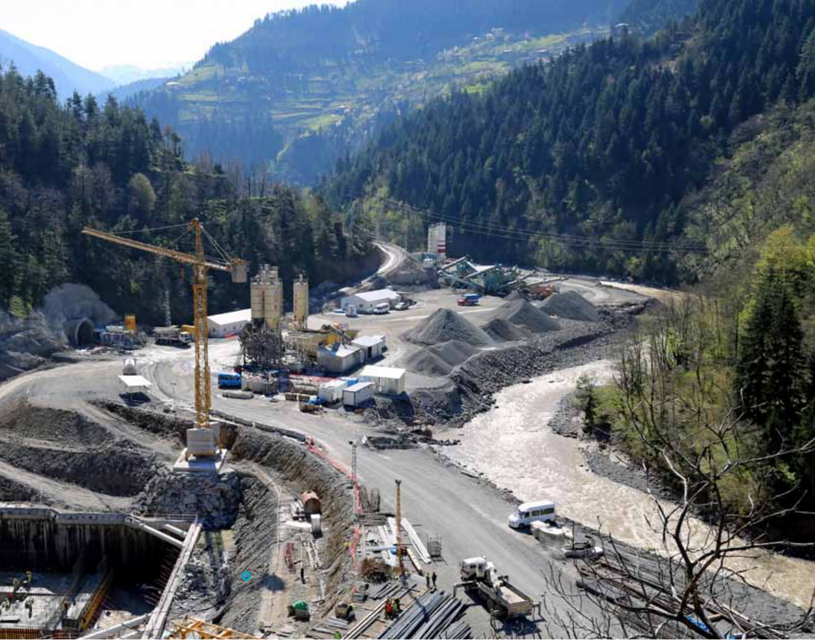
Overview of the project site: The photo shows the intake tunnel (top center) and the foundations of the main plant facility.
