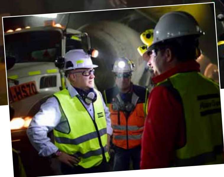
Left, Bjorn Tisell, Atlas Copco, discussing details of the underground access drift excavation with Astaldi managers.
