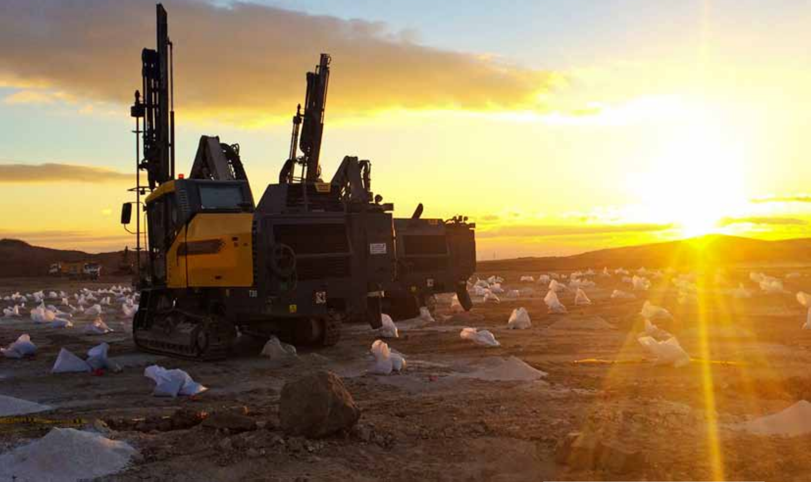
These Atlas Copco SmartROC T35 and FlexiROC T35 rigs were used in the Powerbit test, drilling blast holes 5.5 m in depth. Each rig was equipped with the 102 mm Powerbit T51 with retrac design and spherical HD buttons (right).
