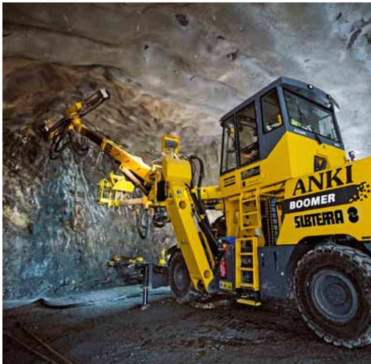
The bypass gets under way: Boomer WE3 in action in the access tunnels.
