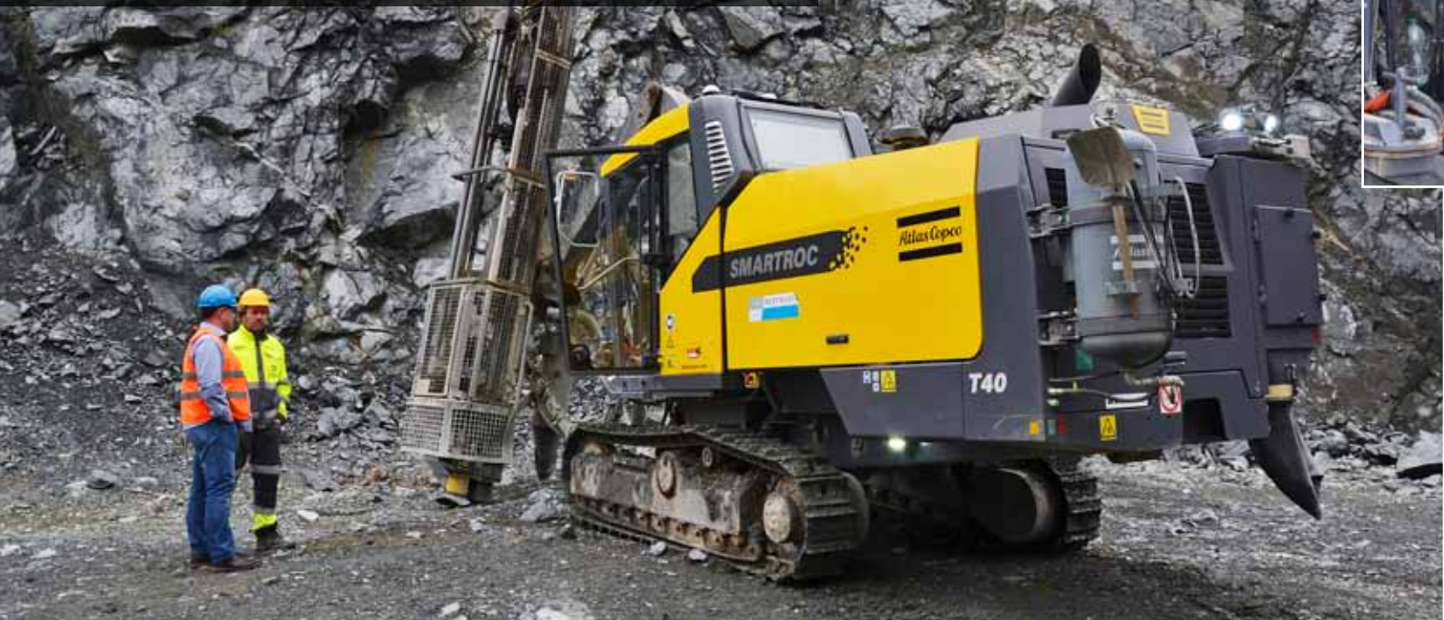
A new SmartROC T40 from Atlas Copco goes to work: Contractor CB Destruckce's CARE agreement means that it does not have to worry about the availability of the machine.
