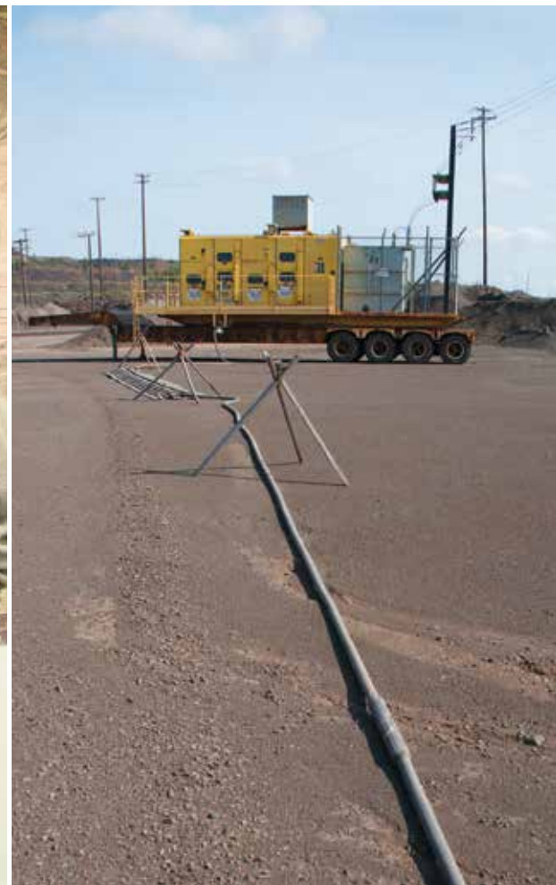
The cost of moving: Moving an electric cable to a new pattern can take hours, and moving the whole rig can take at least a day.
