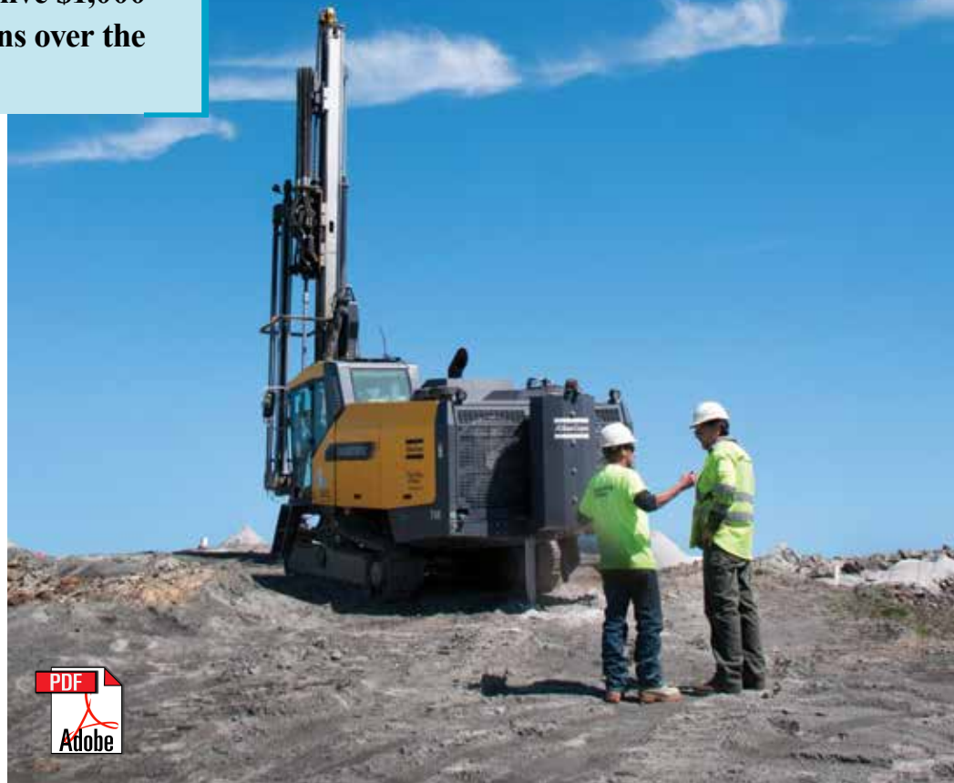
Computerized rigs like this Atlas Copco SmartROCT45, says Executive Vice President Ted Purington Jr., will bring about a revolution in the drilling industry at least as big as the change from pneumatic to hydraulic drill rigs.
