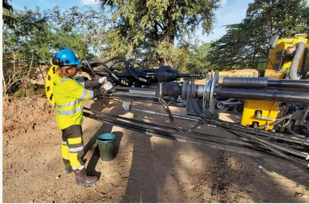
The PowerROC T35 tophammer rig helps the Rapid City Realty and Development Corporation achieve great things in Eastern Rizal in the Philippines.
